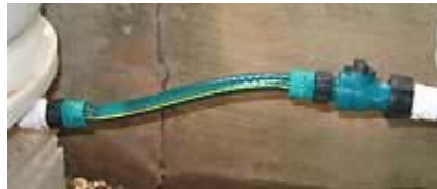
The second rain barrel must be below the first so the rain barrel can drain from the higher to the lower one.
